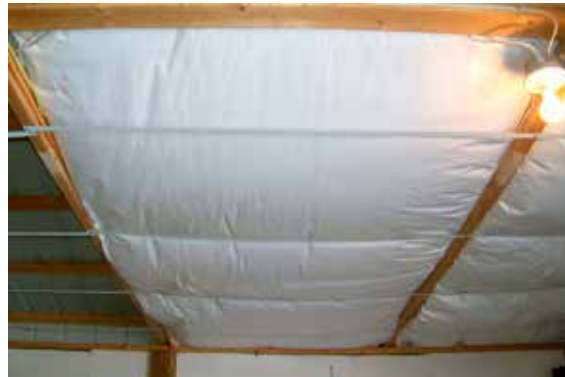
STEEL BANDING Used On Ceiling
